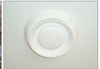
Finished installation with Primex WG Series Diffuser
